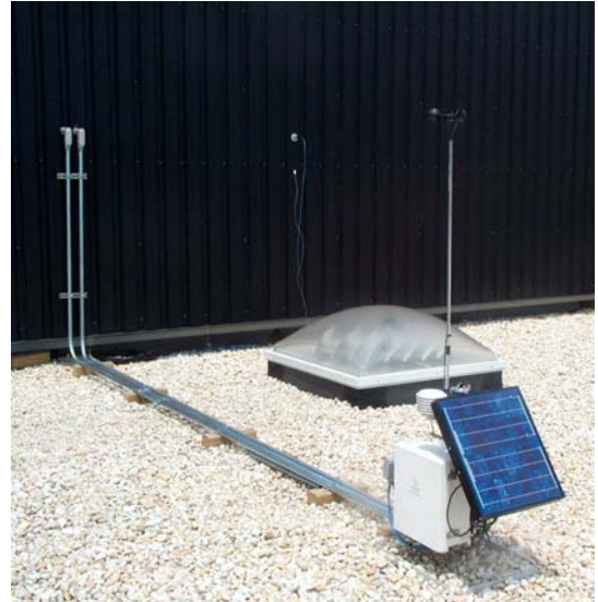
Figure 3.2.1 (above): Warm air distribution duct with sensors to measure air flow and temperature. Figure 3.2.2 (right): Data acquisition system with transpired collector in background.
