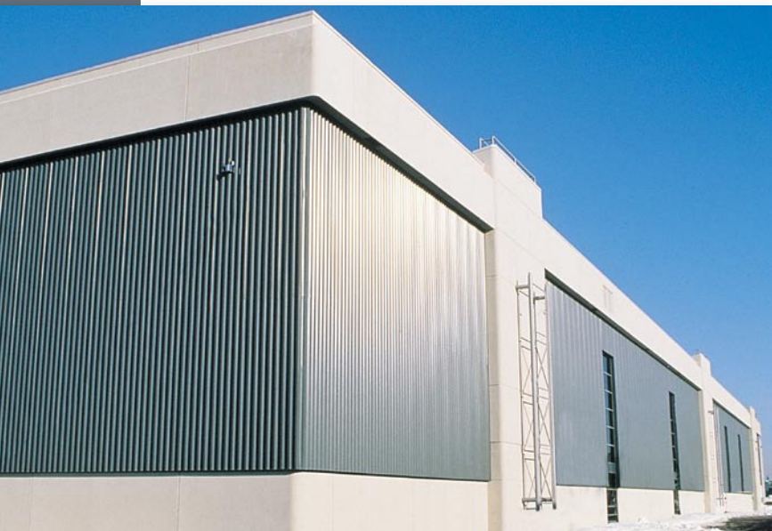
◀ Canadair division of Bombardier: 100,000 ft 2 SolarWall – world's largest solar air heating system.
