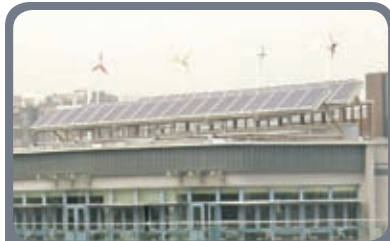
SolarWall PV/T™ rooftop system installed in the Beijing Olympic Village.
