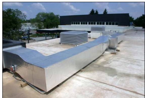
Photo of the Hibbing Annex rooftop ducting and SolarWall system
