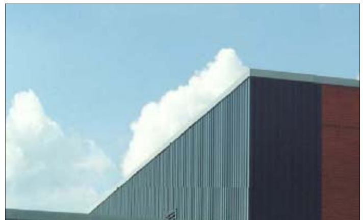
Close-up view of the SolarWall system on the south wall
